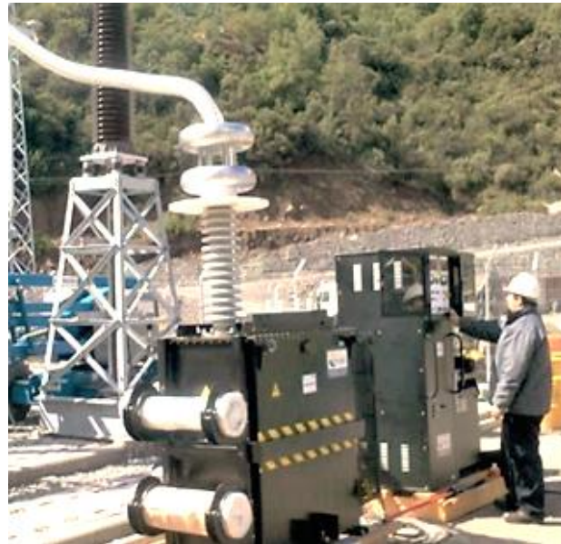
200 kVac Withstand of 138 kV
